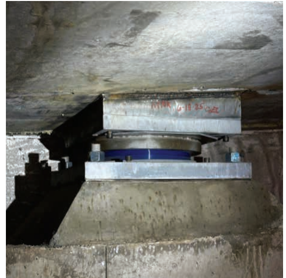
I-70 West Vail Pass Auxiliary Lanes High Load Multi-Rotational Disc Bearing Installation.
